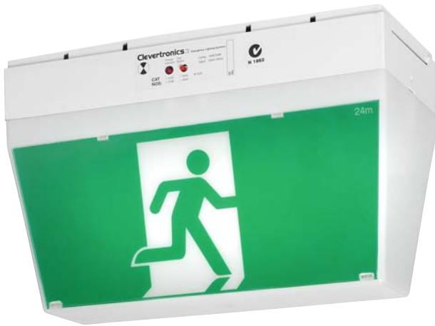
Ceiling mounted Boxlite™ exit
